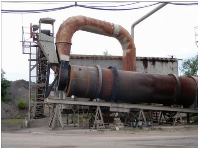
Figure 23. The dryer in a batch-type hot mix asphalt plant heats and dries the aggregate. Also shown: conveyor for aggregate feed (left) and baghouse (rear). Courtesy Northern Bituminous Mix, Inc.
