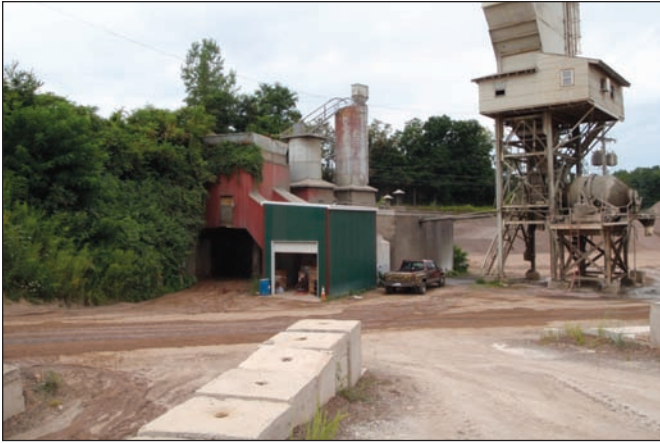
Figure 28. Batch (left) and central ready mix concrete plants. Courtesy Northern Ready Mix, Inc.
