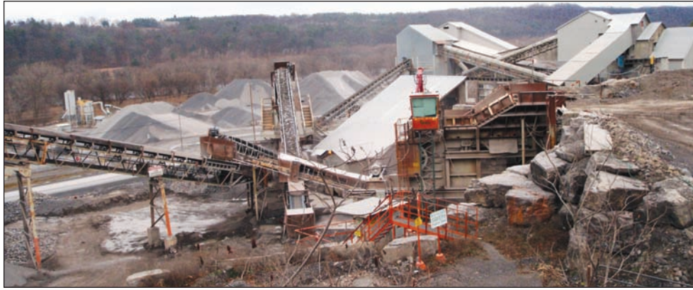
Figure 17. Typical crushing and screening operation. Primary crusher (right) feeds material to secondary crushers and sizing screens. Material is stockpiled by size (background).
